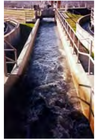
Expand Image The United Water New York wastewater trough.
